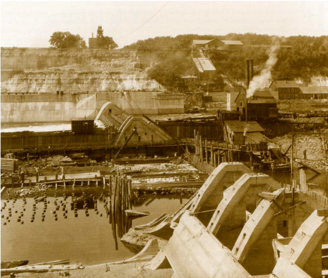
Lock and Dam No. 1, showing innovative prefabricated design that allowed for cold-weather construction, nearing completion, 1916
