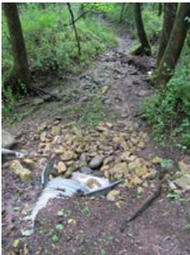
Photo 1. Erosion at culvert, GPS 12. 6-15-12
