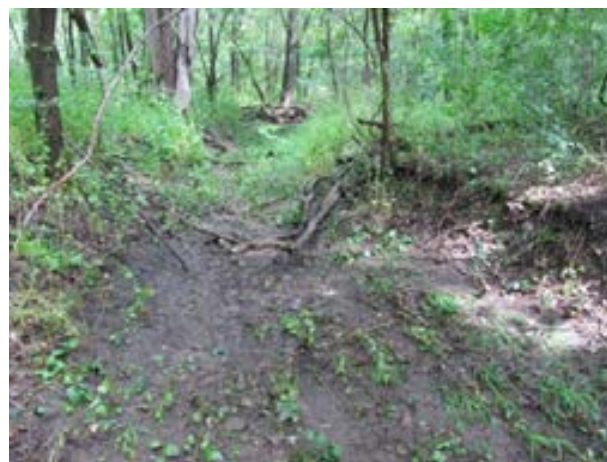
Photo 3. Erosion in floodway. GPS 11. 6-15-12
